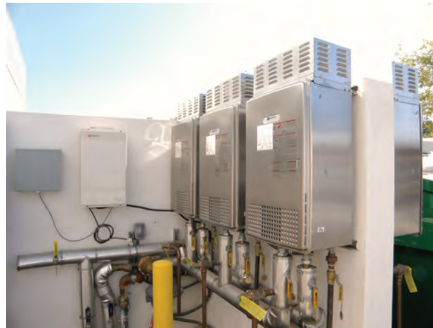
Six units on the ground level providing hot water for the spa and restaurant.
