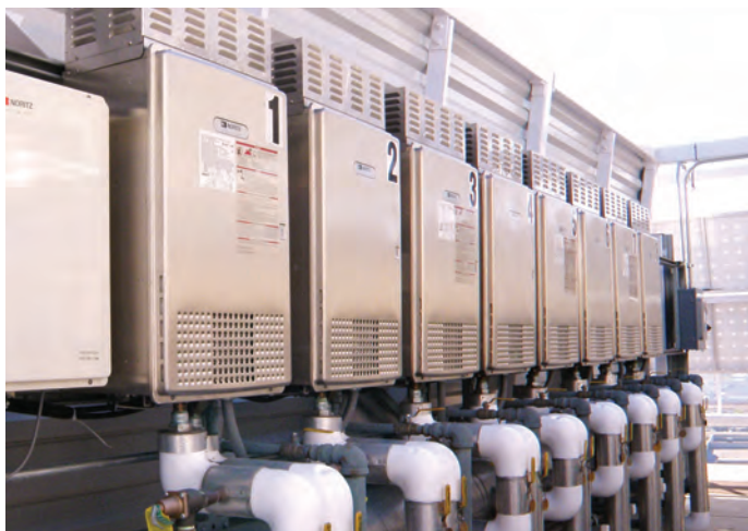
Eight Noritz N-1321M-ASME commercial water heaters on the roof top for 208 guest rooms.
